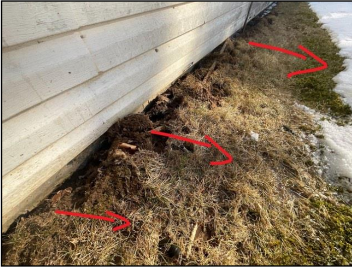
32. Grade should be sloped away from foundatio...
