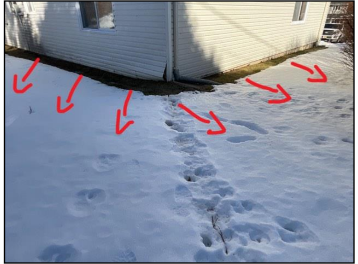
33. Grade should be sloped away from foundatio...
